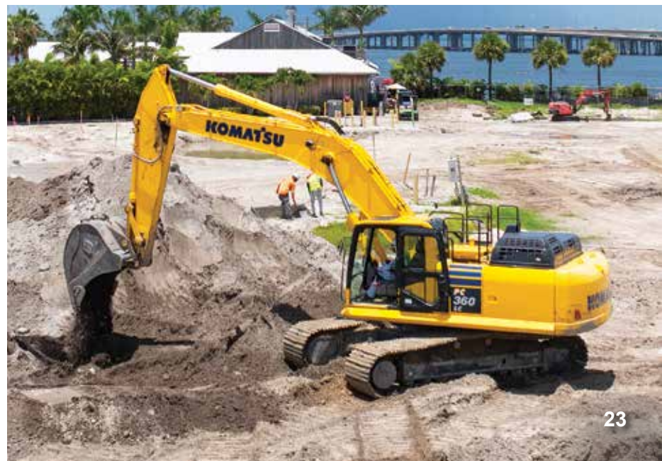
An operator uses a Komatsu PC360LC-11 excavator to place material at Sitecrafters' multifamily jobsite.
