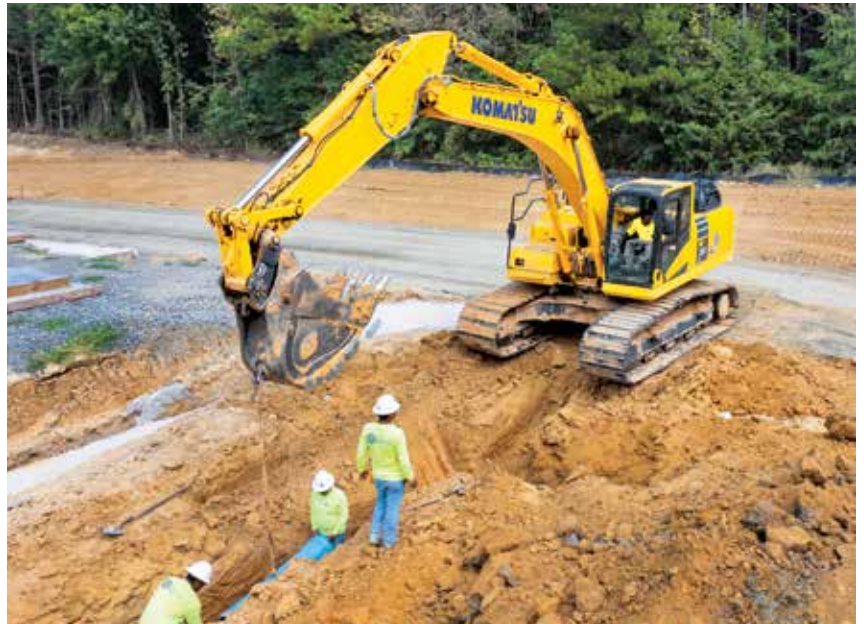
To lay pipe and cut trenches, Elite infrastructure Group relies on its Komatsu PC360LC excavator, which is equipped with a quick coupler for easy attachment changes.
